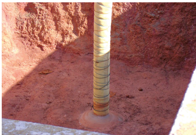
Deep recharge bore well
